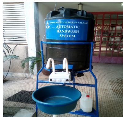
Figure 6: Automatic Handwashing Machine on site.
